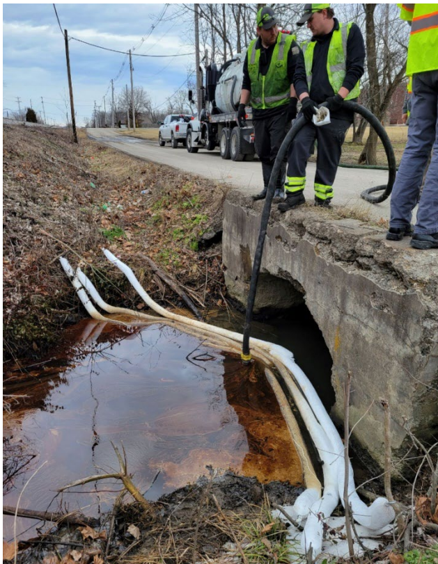
Figure 3 Love's Travel Center Storage Tank Leak
